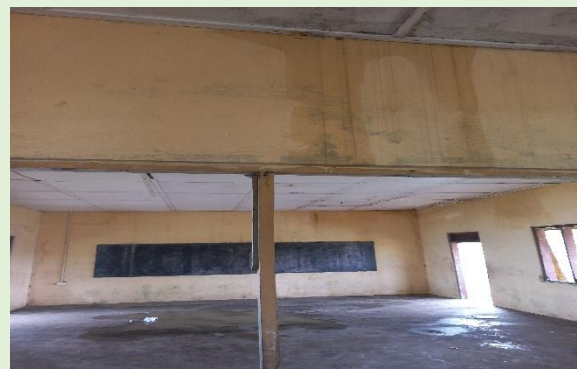
Leaking roof yet to be repaired
