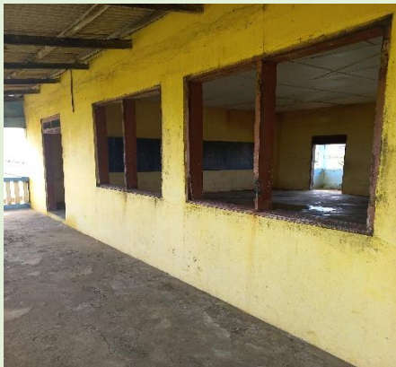
Classroom doors and windows yet to be replaced
